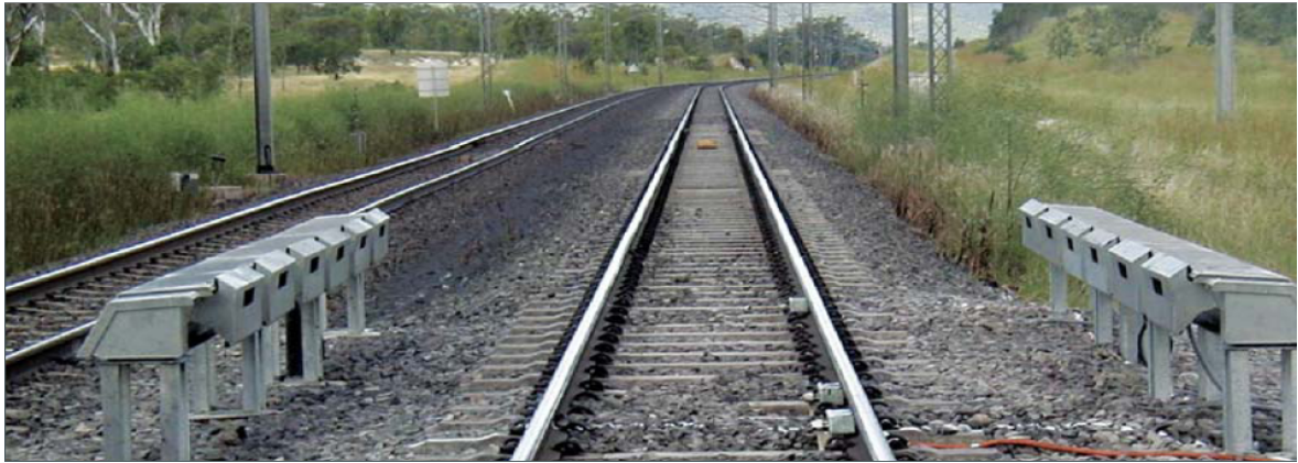
Figure 4: Trackside Acoustic detektori (TADS)
